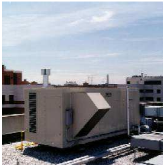
Fig. 8. A Desiccant Unit Atop the Park Hyatt Hotel, Washington D.C. (Source: National Renewable Energy Laboratory, DOE)
